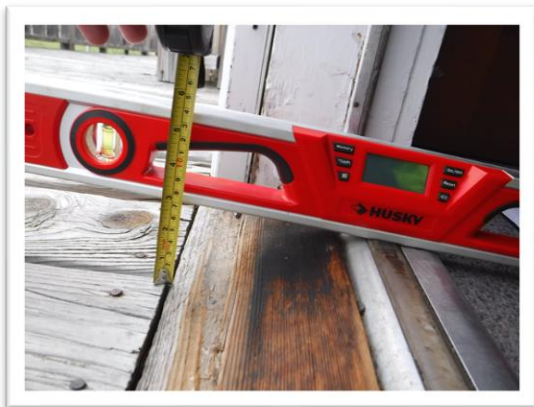
Figure 6: Lobby Threshold (Approx. 3" Above Ground)
