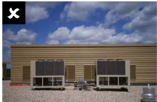
Unshielded roof-top equipment
